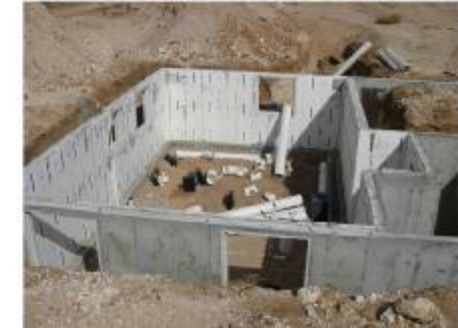
BELOW SLAB DUCTING
